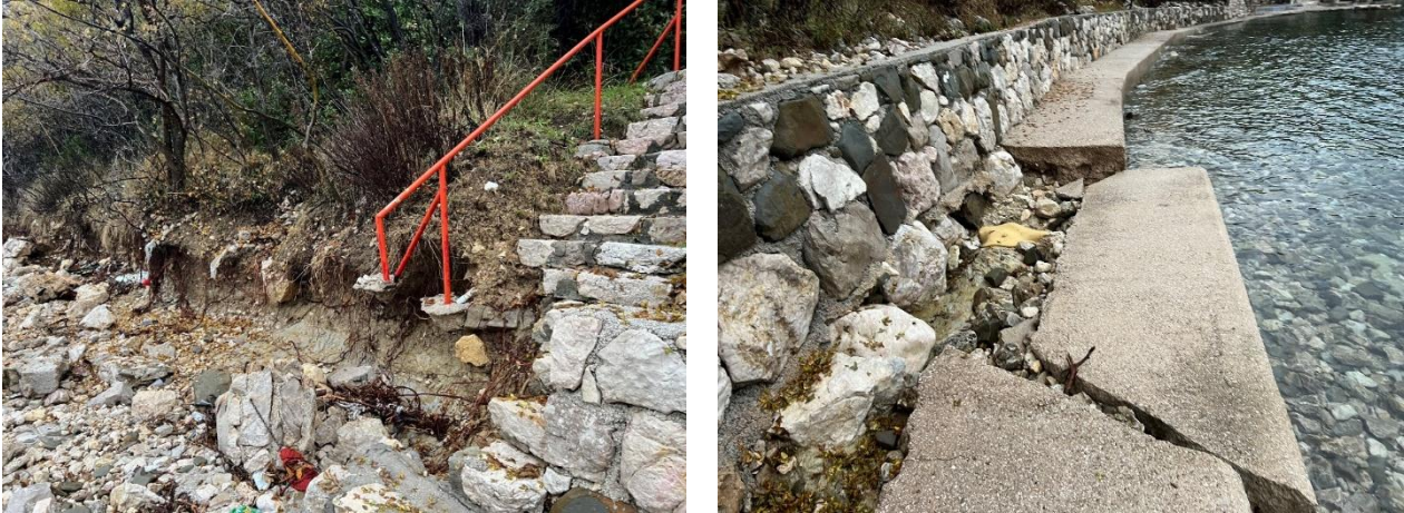
Figure 36 - Examples of past local instabilities at the sampling location due to the slope's toe erosion.
