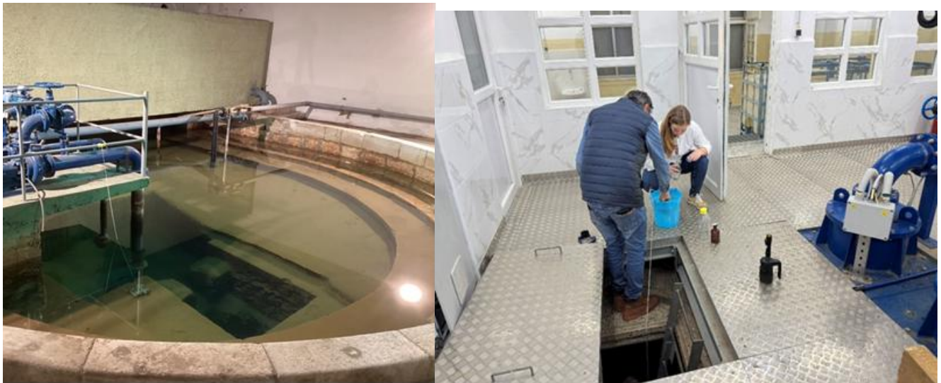
Figure 9. Pumps at Spring Carolina in Pula and at well Tivoli
