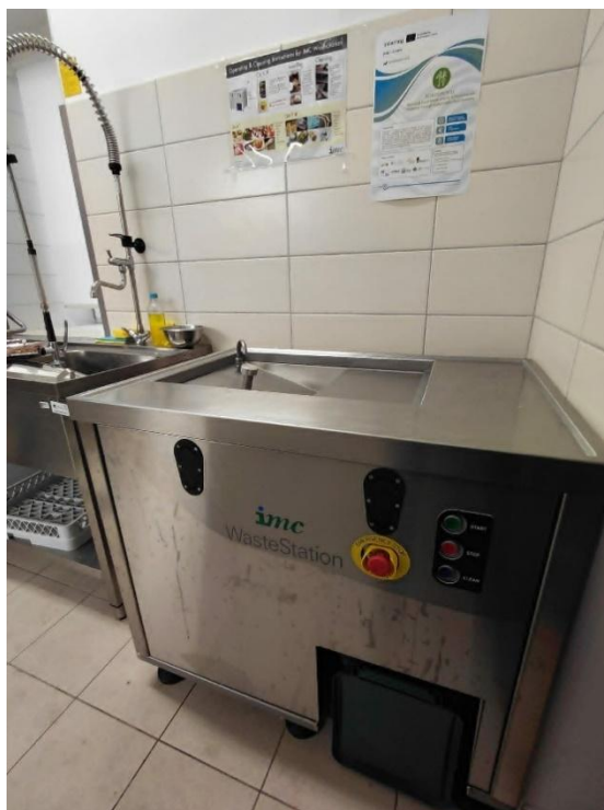
Figure 1. Food waste processing device installed within the school kitchen environment of the Commerce and Catering School Karlovac
